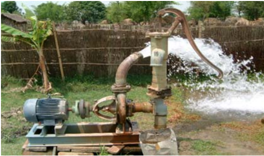
Pump near power plant
